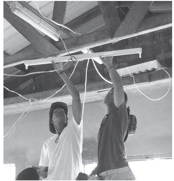
Davice Haugabook '12 and K-Cee Pinkett '14 putting the finishing touches on the electrical wiring at the church
